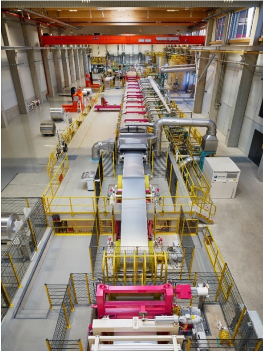
Image 1: The new surface treatment line is designed for a large variety of products. (©AMAG)
